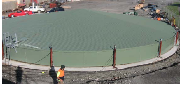
Photo Left: External view of the tank roof and the attached ladder & ladder platform
