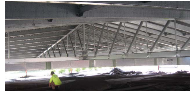
Photo Right: An internal view of the tank roof construction. The special liner is being positioned for our crew to begin the process of attaching it to the roof of the tank.
