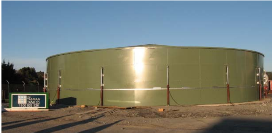
Photo Below: View of TS600 Circular Liner Tank with our hydraulic jacking system being utilised.
