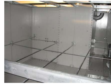
Photo Far Left: Internal View of Tank & Fittings
